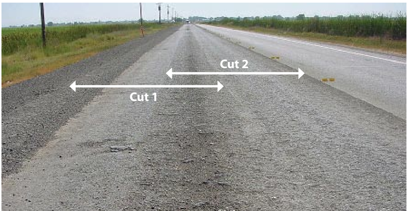
Figure 6.6 Bitumen Starvation along Longitudinal Joint
